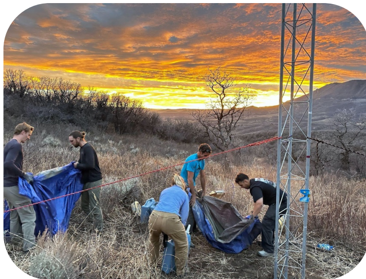
CMC, CW3E, and YVSC team members work together to install a tower at a Y-BASIN station deployment in 2023. Image Credit: Ethan Morris.
