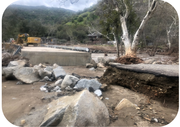
Tulare County crew repairing the bridge after the flood abated. Image Credit: Julia Goolsby.
